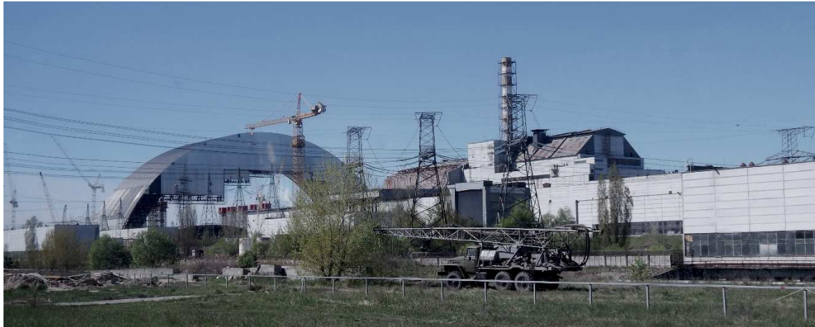
Construction of new confinement for unit 4 at the site of Chernobyl nuclear power plant. Photo: NECU archive
